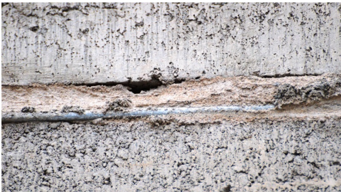
HJR installed without minimum cover requirements
