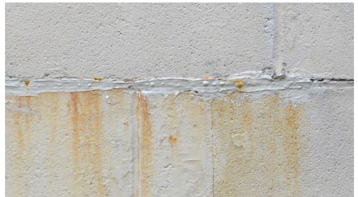
Corrosion of HJR without minimum cover.
